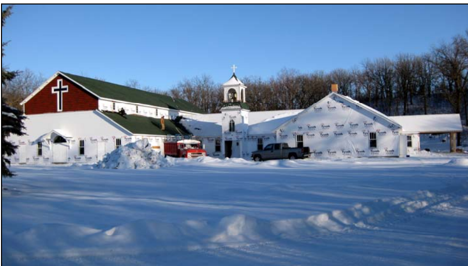
The chapel project as of January 29, 2009. Two men are roofing on the lower west corner of the chapel.
